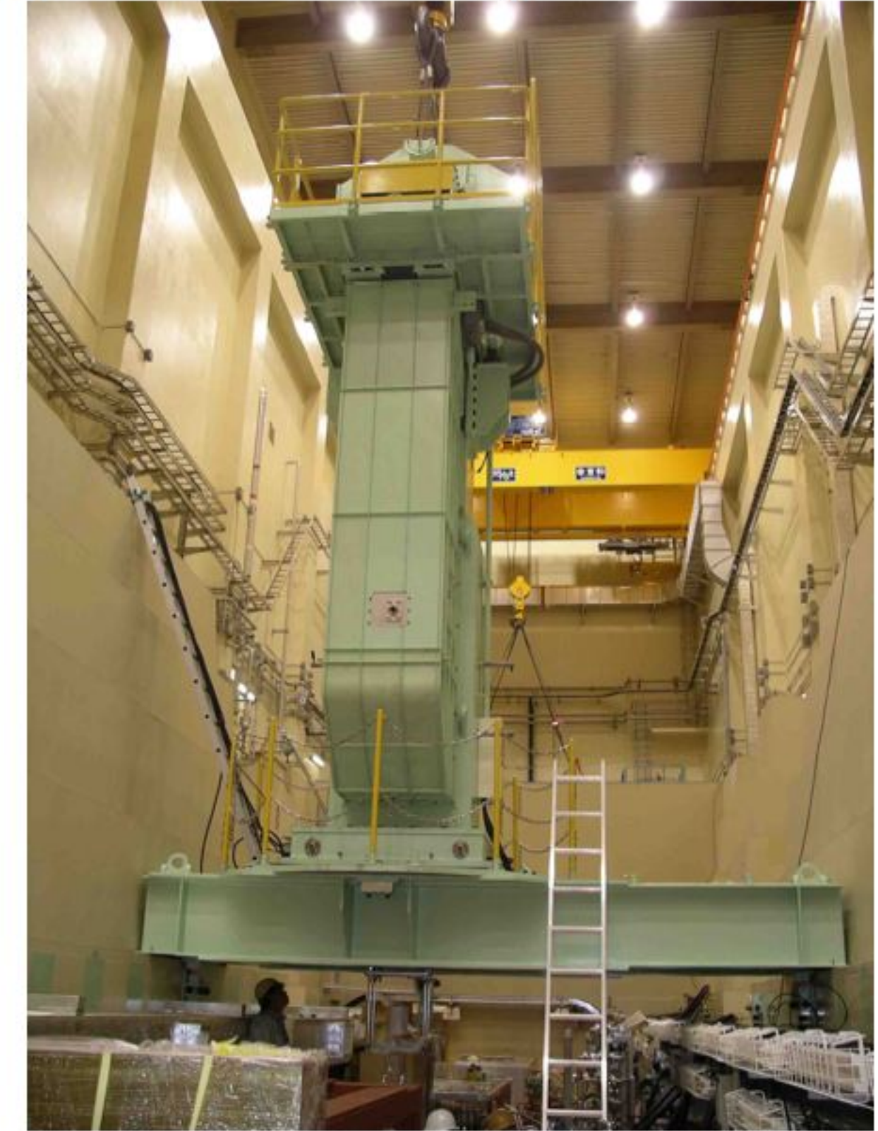
Target cask for remote Handling (transport to hot cell)
